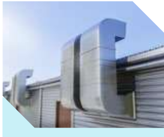
Ducts and Chambers
