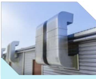
Ducts and Chambers
